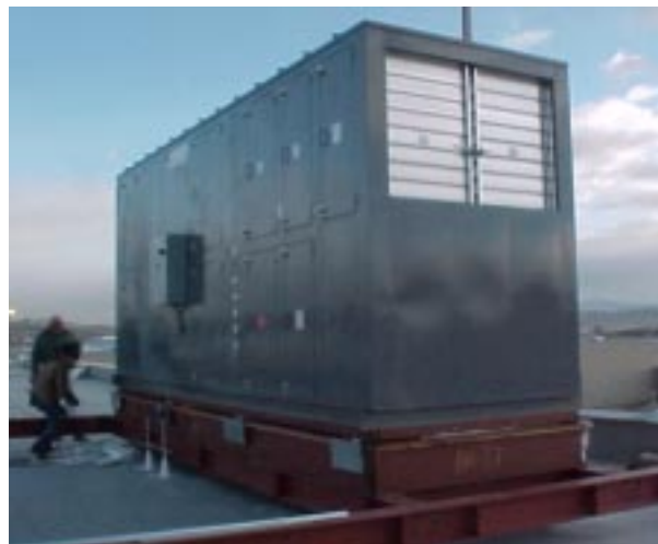
Circul-Aire TMP-15000 unit on airport roof
