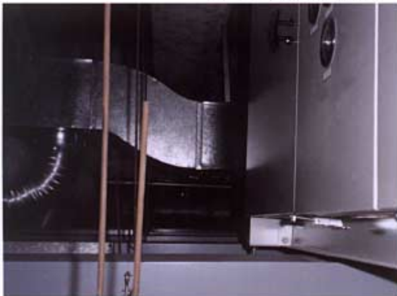
A.P.S.-1500 installed in existing ceiling space of Autopsy Room
