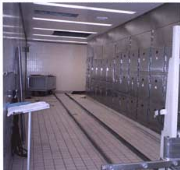
A.P.S.-1500 prior to installation in Main Body Storage area
