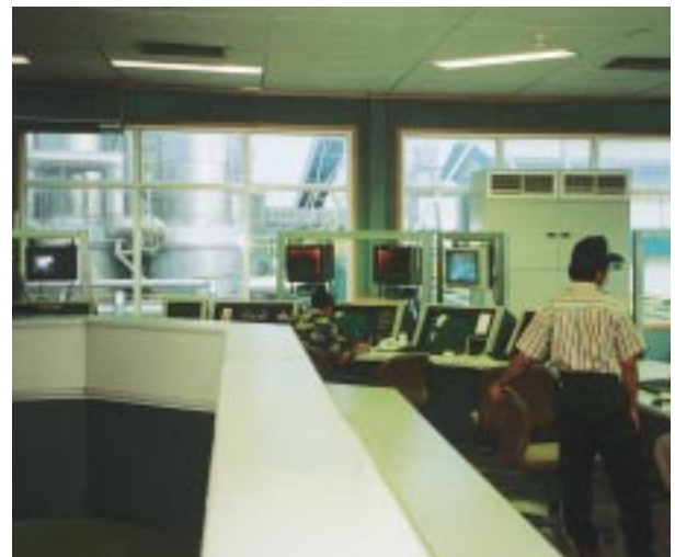
Main Control Room
